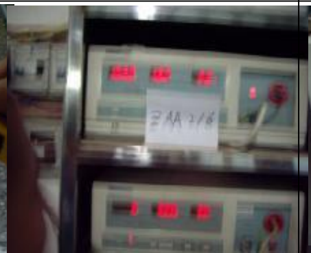
High voltage Test
